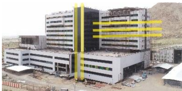
Figure 5.6. View of Qom Noor Heart Hospital
